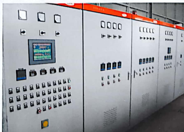
FC001电器控制柜 FC001 Electrical Control Cabinet
